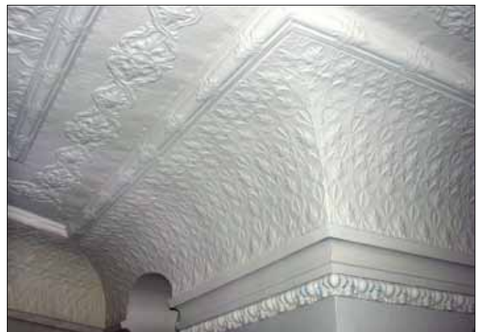
Beautifully crafted tin ceilings and couve moulding around the top of the Town Hall auditorium.
