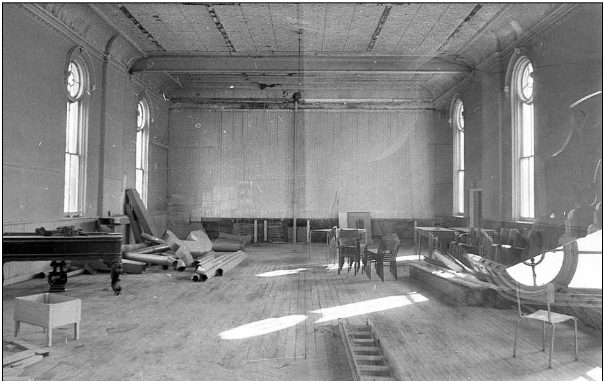
This picture shows the condition of Town Hall 1873, about a year after work began on renovating the century old hall.
