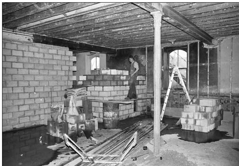
Work got underway restoring the basement of the Town Hall in February 1975, including a new floor, cement block walls and steel support beams under the floor.
