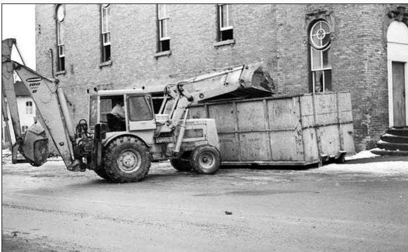
The Town Hall 1873 was undergoing considerable activity throughout December 1974. After a thorough clean-up a couple of weeks ago, workman have moved in and broken up remnants of the old concrete floor and are making it ready for a new floor to be poured. In charge of the work is Mr. Dale Procnier, assisted by two local boys, David Litt and Randy Jobin.
