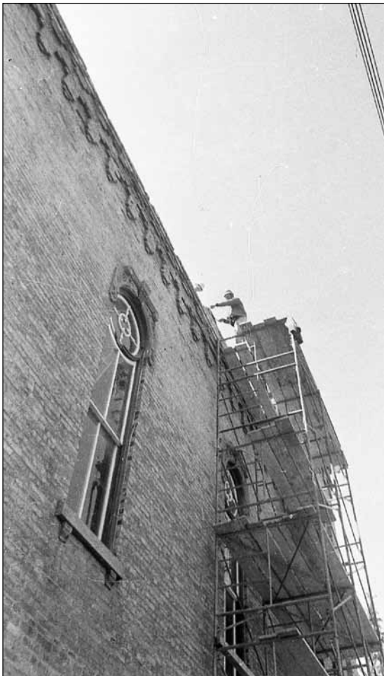
Construction inside the Town Hall had been steady all winter and now that spring has arrived repairs to the exterior got underway. Martens Masonry & Construction Ltd., commenced the work of repairing and replacing the brick parapet on top of the building. April 14, 1975,
