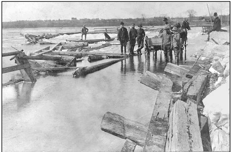
Workmen begin repairs to the Scugog Bridge after ice damage in Spring of 1908.
