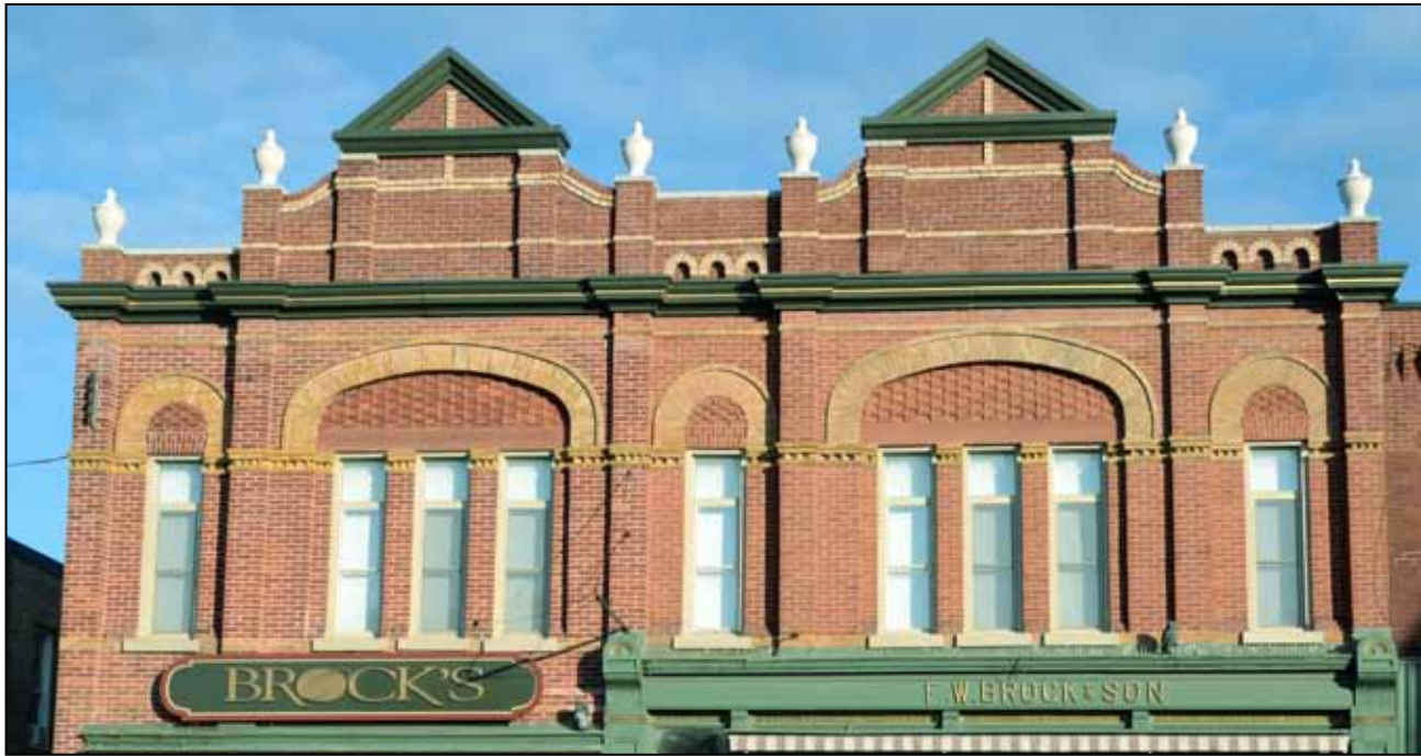
The familiar Brock block, which had been without parapets for almost a century, had them replaced in 2018.
