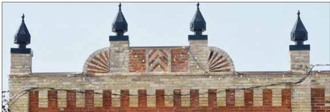
Re-built parapets on the top of the MacIntyre building, at 235 Queen St., Port Perry
