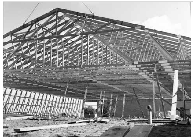
The new Peel's Hatchery in 1966. Trusses and construction of the plant was done by Lake Scugog Lumber.
