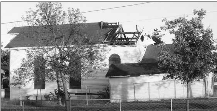
Damage to the fair exhibit building after the destructive storm of May 2018.
