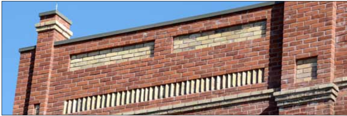
Major repair work on brick and parapets took place on the Lattrielle and Puckring block in 2013.
