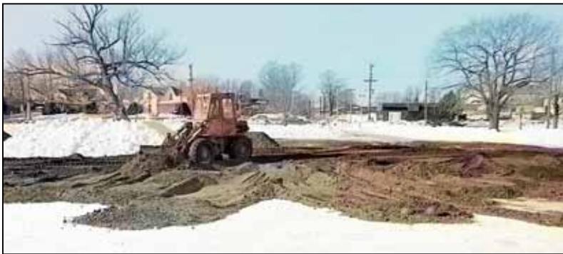
Above: Work gets underway, dumping sand onto Lake Scugog ice, in February 1979.
