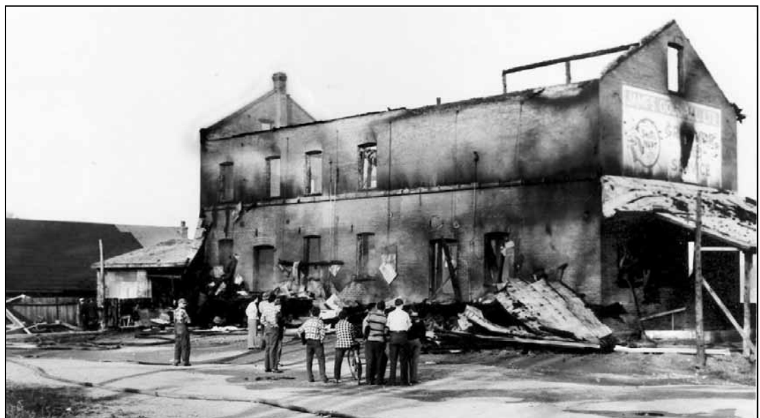
Residents gather around to survey the burned-out shell of the James Goodall building following the fire.
