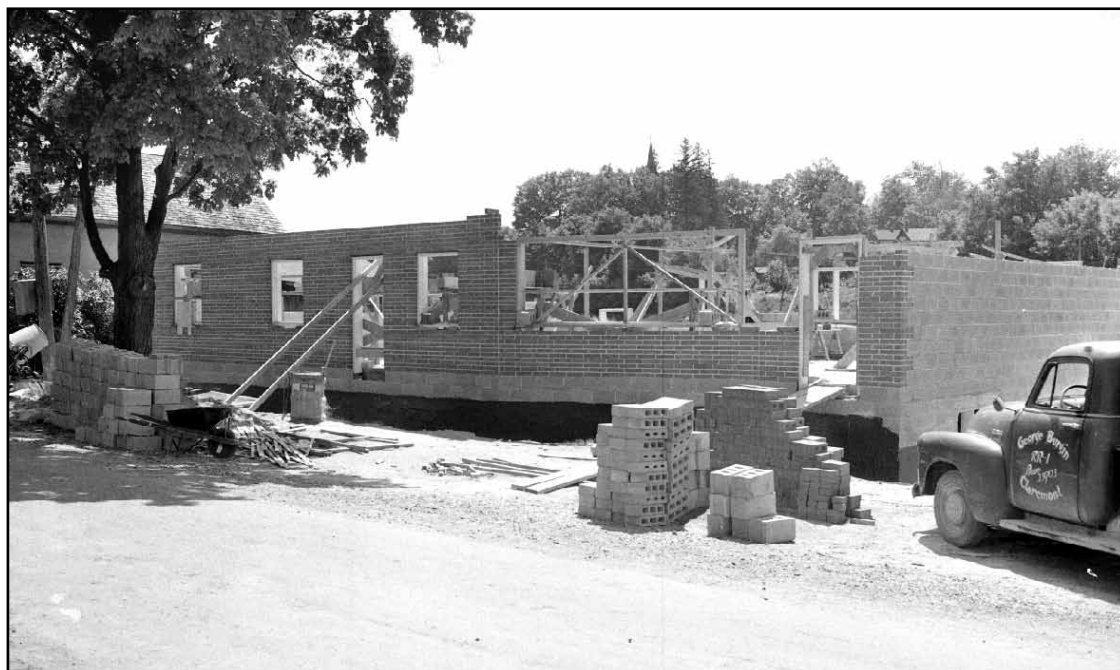
The new Uxbridge Times-Journal on Bascom St. is seen during construction in 1957. The building was completed and formally opened in November 1957, with Mayor Carl Puterbough cutting the ribbon for the official opening.
