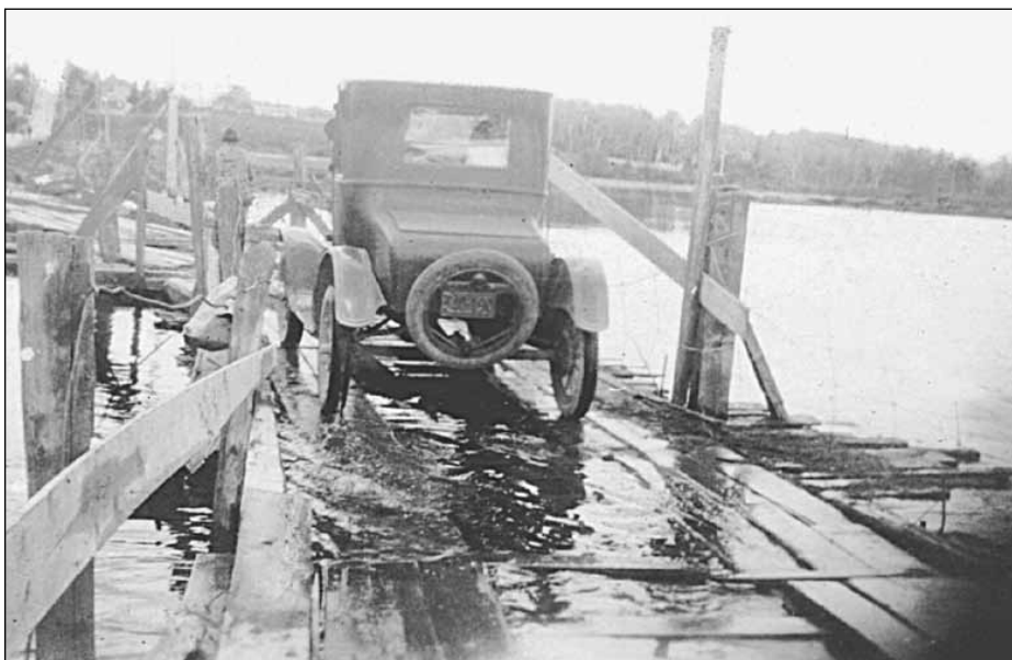
A car carefully makes its way across the floating detour used during construction on the bridge.
