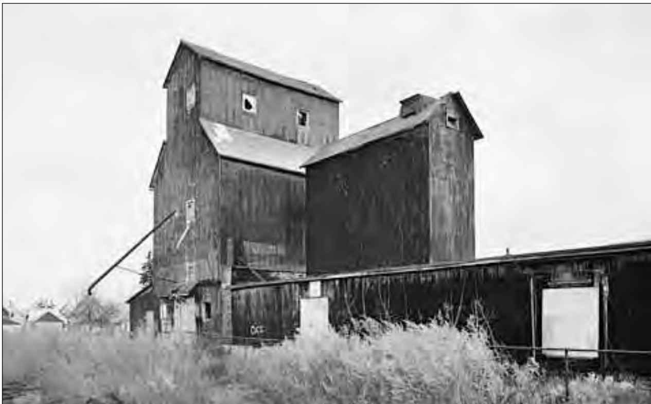
This picture is of the Wollenberg Grain and Seed Elevator, Buffalo, N.Y. Due to its similarity to the Port Perry Elevator, it was used as a reference for some of the technical information in this article.
