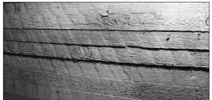
Stacked 2"x 8" bin boards.
