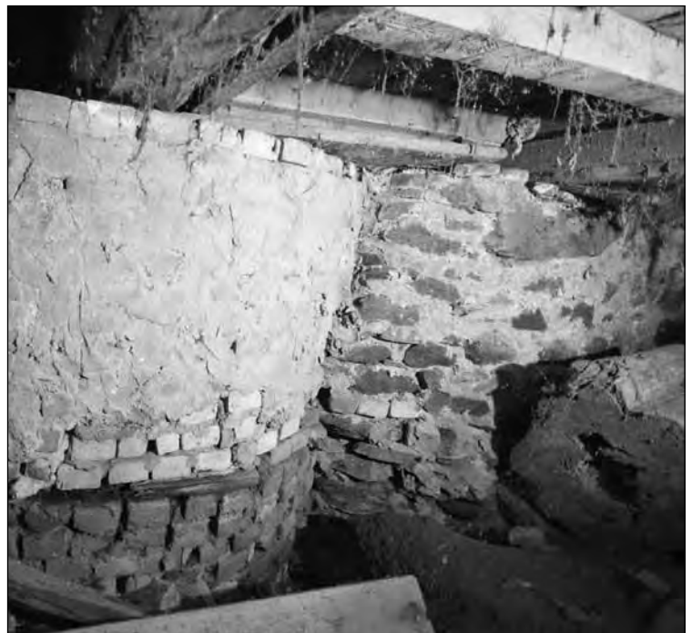
The foundation of the elevator was originally stone, but appears to have been repaired a number of times with brick and cement patching.
