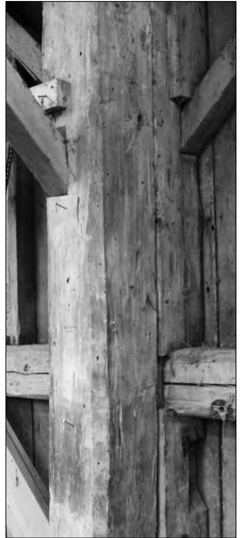
Huge posts and beams, some as large as 10"x 10" in size, helped provide the strength of the structure.
