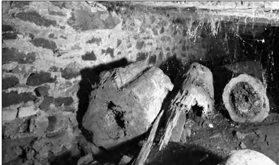
Huge wood support beams now rest on the dirt floor, beside the original stone foundation, having been replaced by concrete piers.
