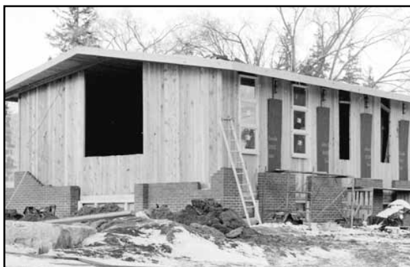
The new Baptist Church at Rosa and Queen St., Port Perry while under construction in December 1963.
