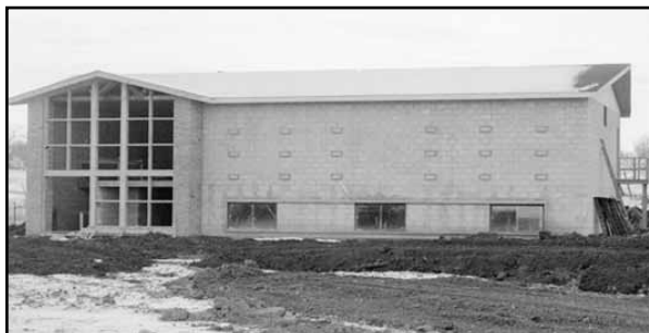
The new Oddfellows Hall, south of Port Perry during construction in December 1963. The hall was officially opened in June 1964.
