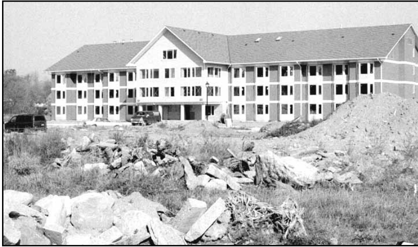
Problem plagued West Shore Village complex, on Simcoe St., into third year of construction.
