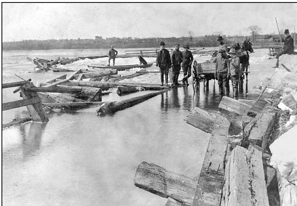
Scugog Bridge was damaged by ice during the spring thaw in 1908. Photo shows ice damage to the upper cribbing and railings. Men on bridge are Ben Pettit, second left, (grey whiskers). Geo. Jackson next to Ben and Sam. Wakeford in boat. Others are unknown.
