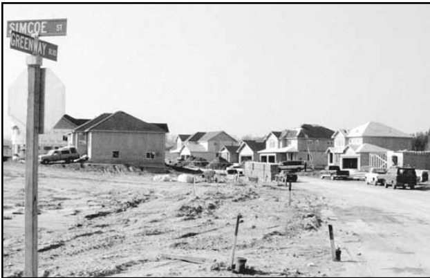
Construction gets underway on "Seasons" a subdivision being developed by Alliance Homes, south of Port Perry on the west side of Simcoe St.
