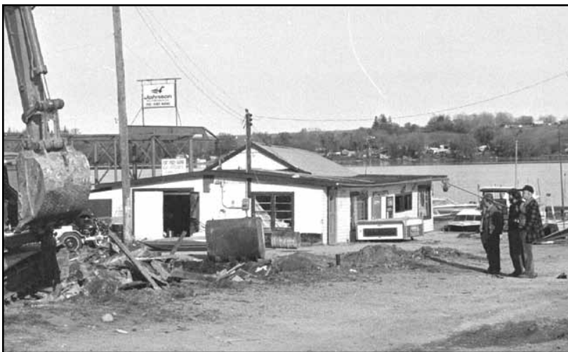
The old Port Perry Marina was demolished to make way for new building in Nov. 1985.
