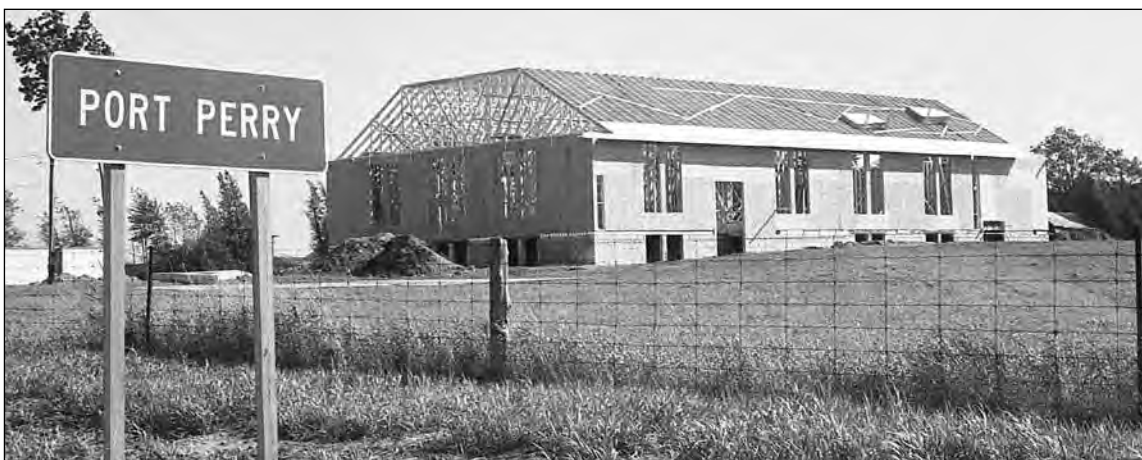
Work on the new Port Perry Pentecostal Church, on Durham Road 8 across from the Scugog Arena, was progressing well in October 1988, with the roof trusses in place. It was only seven weeks ago the congregation gathered at the new site to turn the sod for their new building. Rev. David Beesley and his congregation hope to be able to hold their first service in the new building before Christmas.
