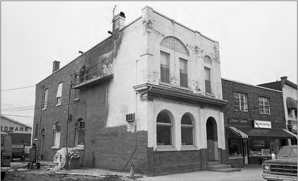
In April 1981, contractors started sandblasting the white paint off the red bricks of the old Bank of Commerce building. The work caused considerable damage to stores in the vicinity of the building being sandblasted.
