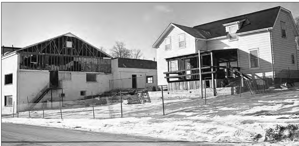
Demolition was underway on the Creamery building, left, and the former Frank Real Estate building, right, in March 1989
