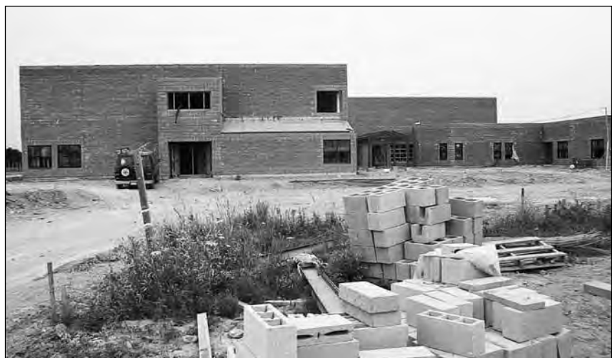
Work on the new S.A. Cawker Public School are progressing and the Board of Education says it will be open for students in September, 1989.
