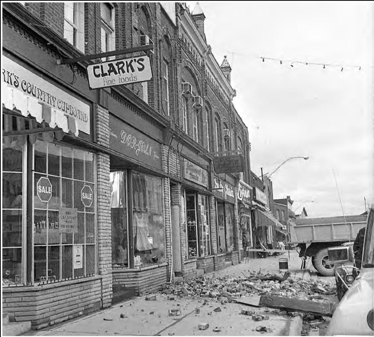
Hundreds of pounds of brick, cement and wood tumbled to the sidewalk on Queen Street in April 1981 after high winds toppled a section of the former Emerson Block, now owned by Tom and Daphne Mitchell. One woman narrowly escaped with her life when the bricks crashed to the ground around her. Township crews were on the street quickly, cleaning up the debris, and the Mitchell's reconstructed the cornice to its original condition.
