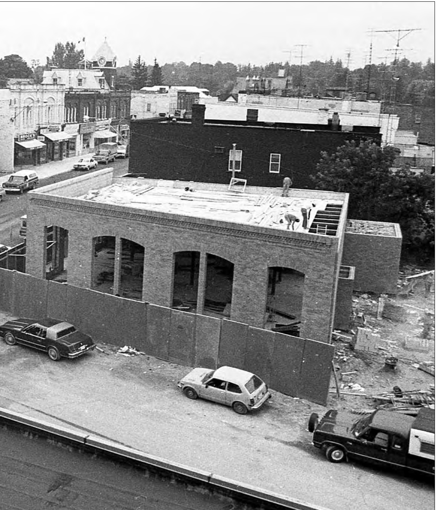
the old Port Perry Arena just to the north (right) of the new bank building, was being torn down (see page 15). Also noticeable in this picture, are the new sidewalks being laid along the south side of Queen Street, in front of the Re/Max office on the corner.
