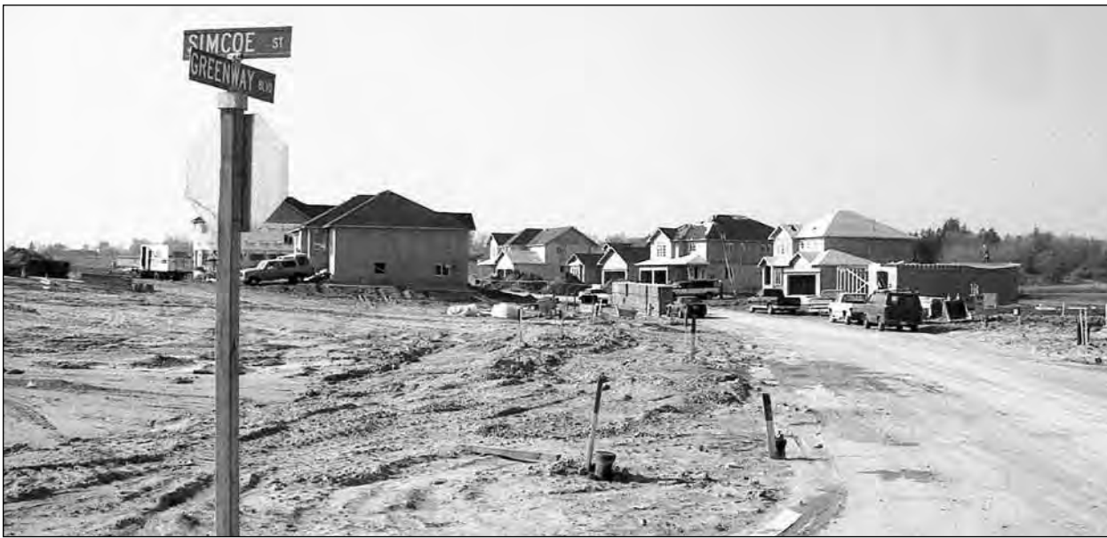
Construction was well underway in October 1998 on a new subdivision, being developed by Alliance Homes, located south of Port Perry on the west side of Simcoe Street.
