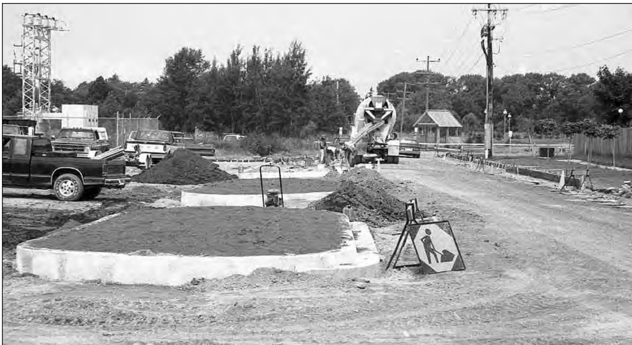
Work was well underway on an $85,000 facelift of the boat launching area in August 1994. The project includes marked parking spaces, islands, curbing, flowers and trees. The new configuration will provide 56 regular parking spots and 23 boat, trailer and bus parking spaces.
