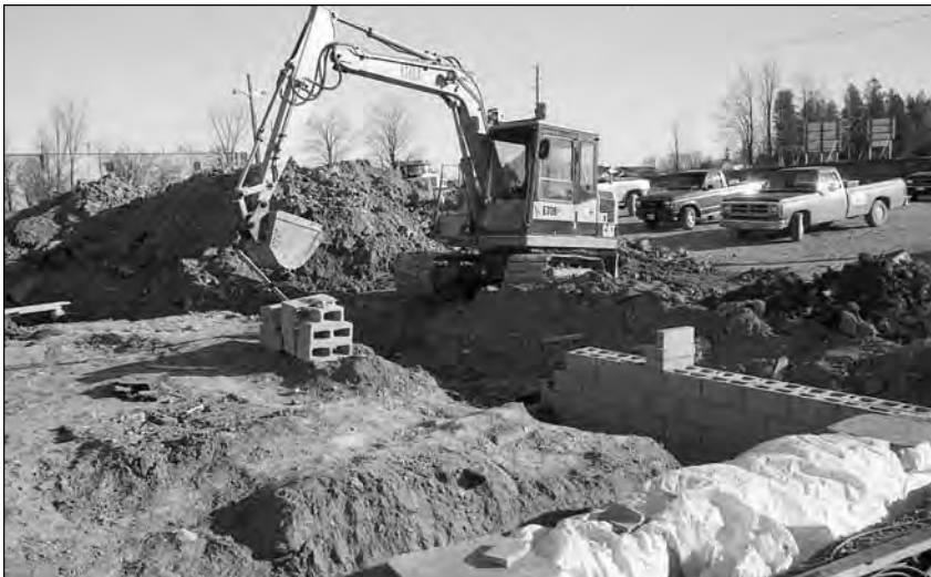
Preliminary site work on Scugog township's new community hall, beside the arena on Reach Street, got underway in early January 1995. The total price tag for the building and parking lot is expected to be about $1 million. It is hoped work will be finished in time for an opening ceremony about May, next spring.
