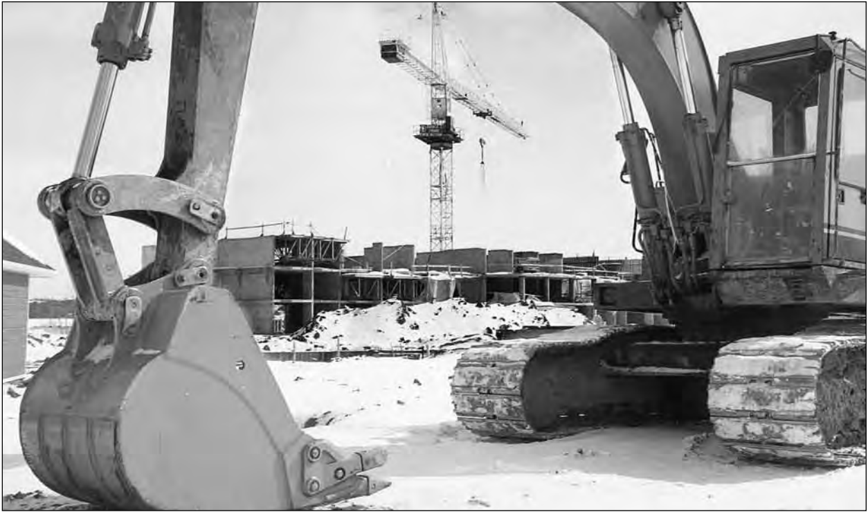
Work on the three-storey West Shore Village complex came to a virtual halt during the winter of 1996-1997, due to delays by planners, engineers and a difficult winter. Developers said there were a lot of surprises encountered when putting in the hard services, such as sewer and water lines due to soil conditions. This photo, taken in March 1997, so the stalled construction site.
