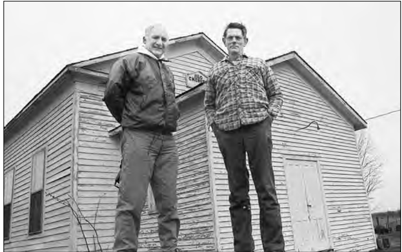
The Head United Church at Scugog Shores Museum Village is in need of a major restoration job which is estimated to cost approximately $60,000. In order to undertake this project, the historical society is conducting a fundraising campaign during the month of May 1993. Pictured above are, left, Paul Arculus, president of the Lake Scugog Historical Society and Jack Kane, a society member.
