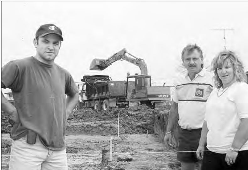
Port Perry will soon have another pool, and an indoor one at that. Donna Kaye, Mike and Steve Cochrane broke ground in May 1998 for what they say will be a multi-use private gym complex on Old Simcoe Rd., next to the Durham Regional Police station. The owners say they hope to set up swim lessons and public swimming times, as well as a fitness centre. No date was given as to when the pool will open, or the name of the new complex.
