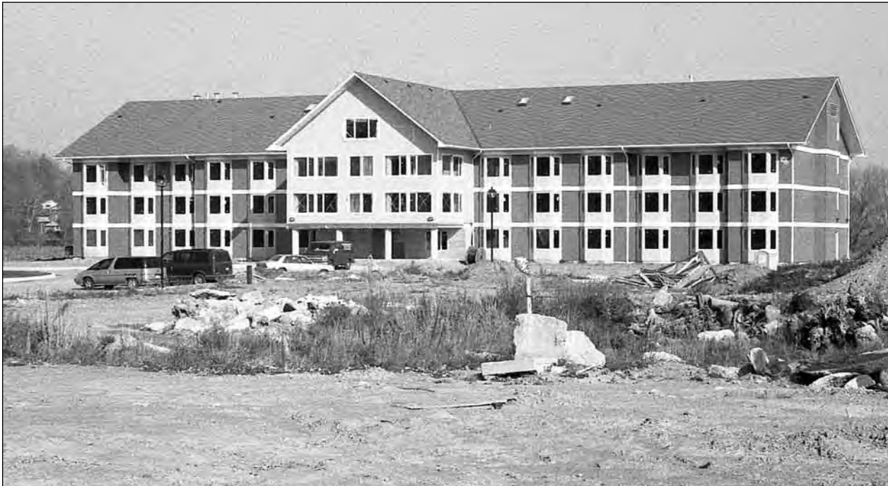
Progress on the West Shore Village project along Perry Street, Port Perry slowed down again in October 1998, as one of the contractors pulled its workers from the site. The project has been plagued by delay after delay since first being proposed March 1995.
