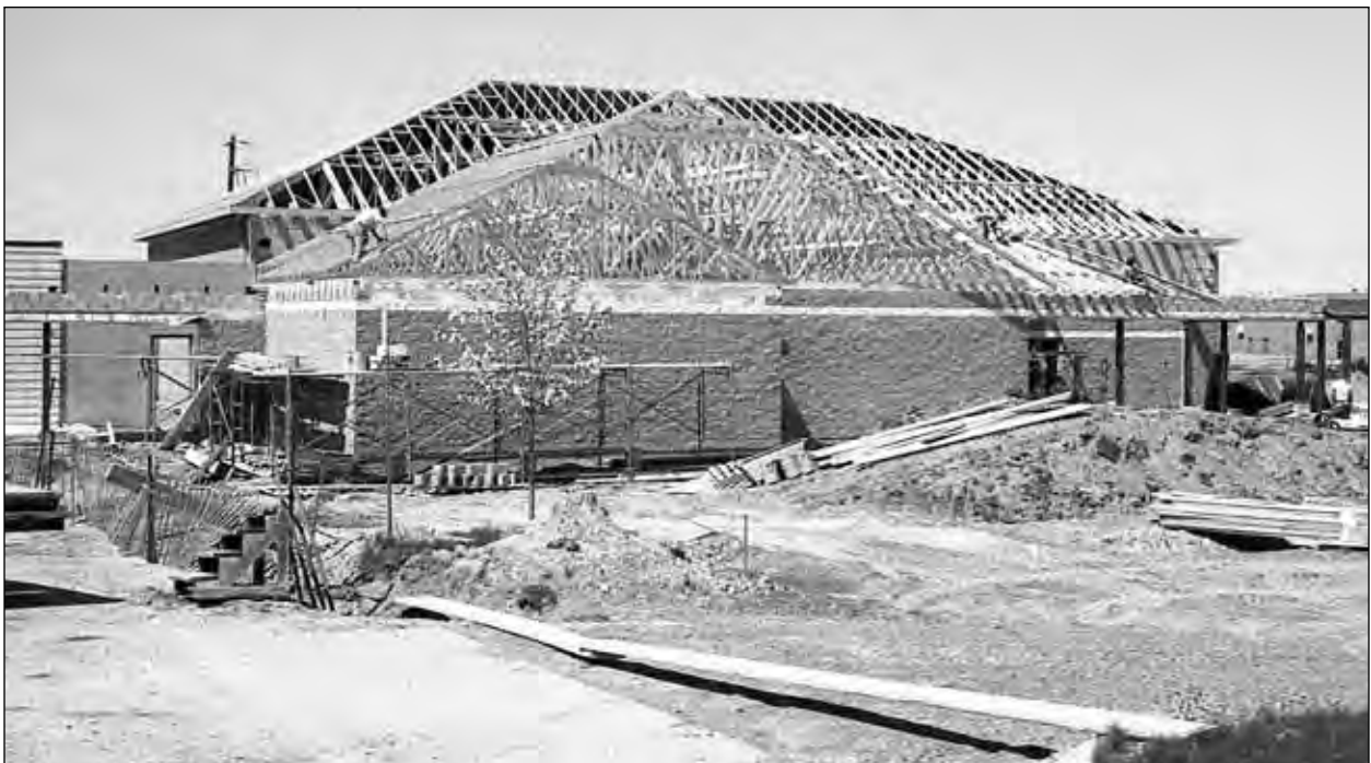
Construction of the Scugog Township's new Community Centre, located on Reach Road beside the Scugog Arena, was progressing favourably in June 1995.
