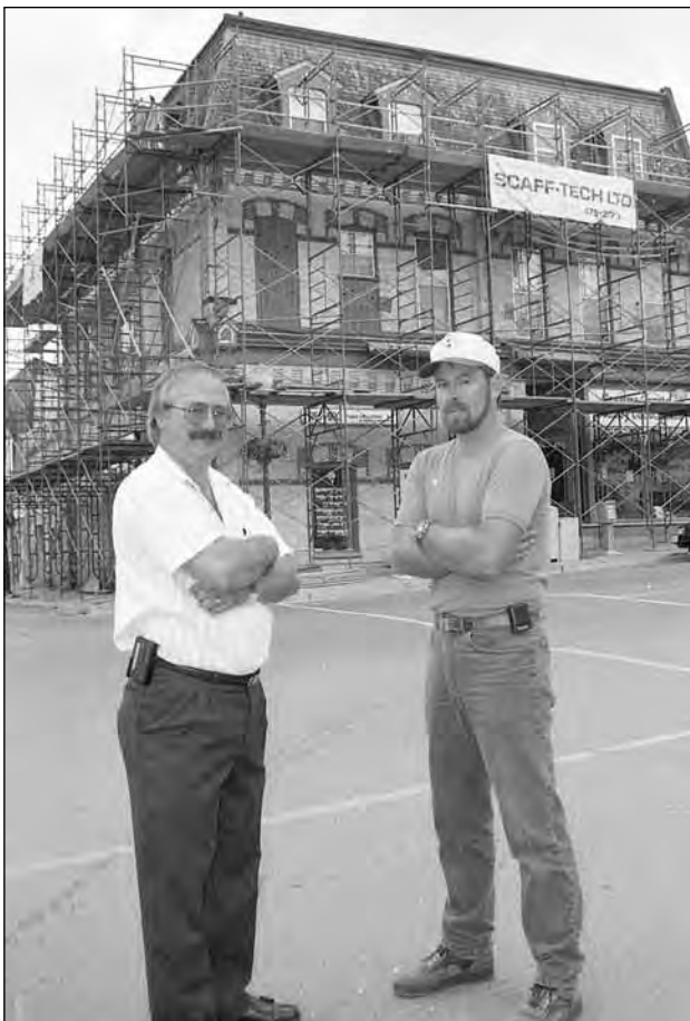
Restoration was well underway in September 1994, on the 110 years old building in Port Perry originally built as the St. Charles Hotel. Re/Max owner Guy Latreille, left, said that restoration of the three-storey structure will cost about $50,000 and will take about a month to complete. Contractor Steve Snider, who is undertaking the restoration, is seen with Mr. Latreille.
