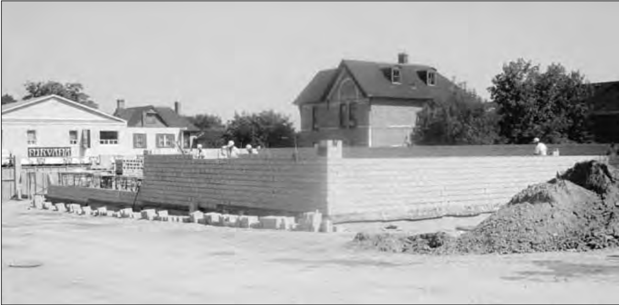
Construction on a new Big V Drug Store, on the former Anderson Chevrolet-Oldsmobile site, was moving along well in August 1993.
