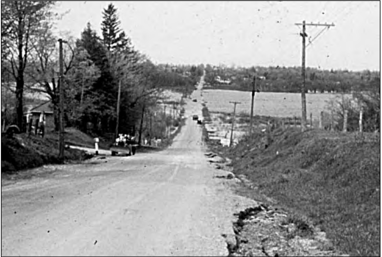
This view from the top of Scugog Island hill, shows the washed-out condition of road on the hill and construction underway on widening and raising the roadbed, further west on the causeway, near Port Perry.
