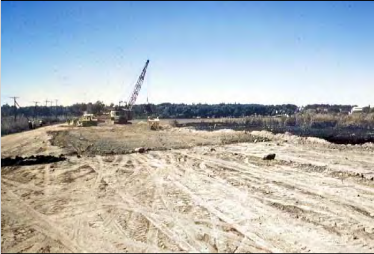
Work is seen, in these two photos, well underway on rebuilding 7A Highway and the causeways from Port Perry to the Caesarea cut-off. The extensive work was completed as scheduled by the government, during 1962.
