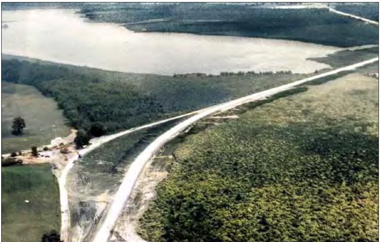
Aerial view of a section of the Cartwright section of the new road being constructed during 1960-1962. The road coming off the Island, bottom left, was re-routed and a new road bed was constructed heading towards the Cartwright causeway.
