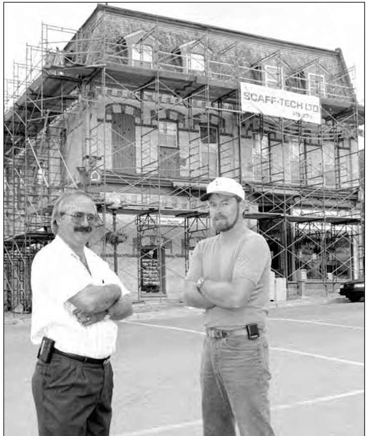
Guy Latreille with contractor Steve Snider during renovations of the historic St. Charles Hotel on Queen St., Port Perry in 1994.
