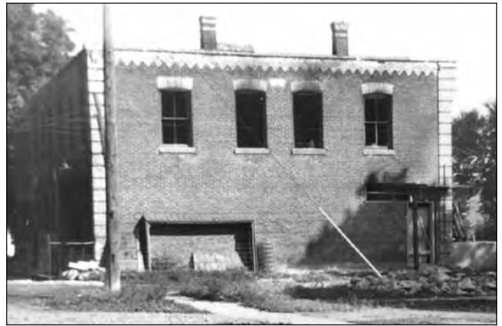
The south end of the burnt-out Morrow Farm building shortly after the fire.
