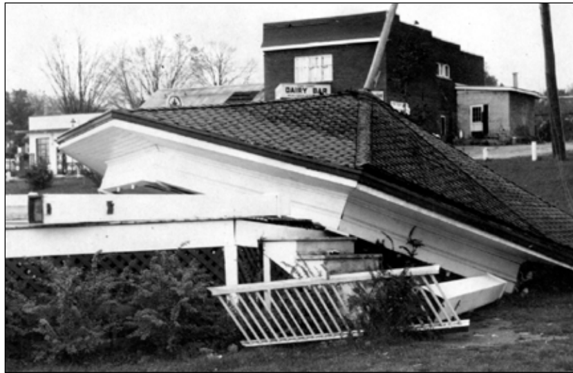
The 25 year-old Band Stand in Palmer Park collapsed during the height of the storm.
