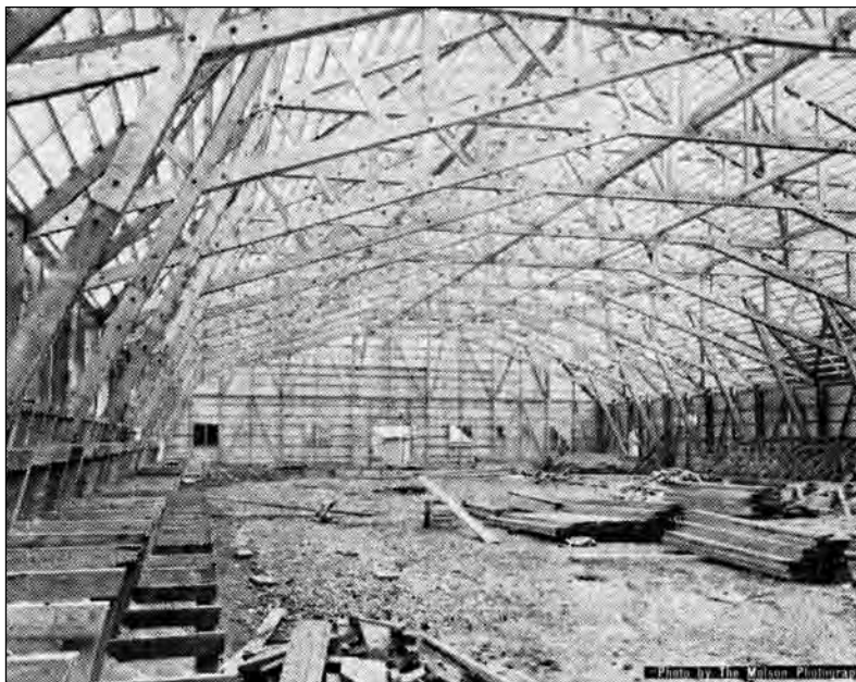
The interior of the new arena shows the truss roof in place and work beginning on the spectator stands. Photo taken in September 1950, by the Molson photographer.
