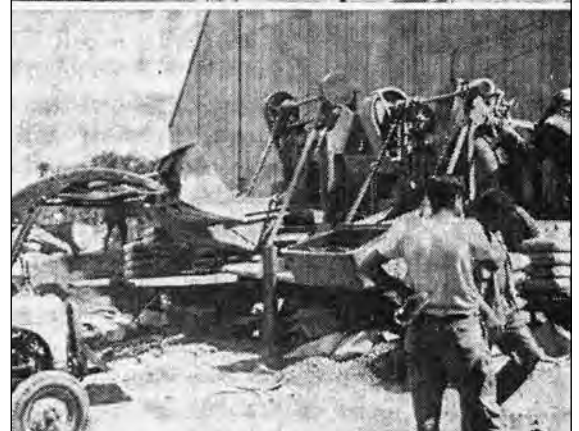
The above pictures show the machinery mixing the concrete at the rear of the arena, and the pouring of the mixture around the pipes.
