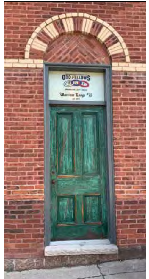
This green door, located on the west side of the Remedy drug store building, at 209 Queen St., was recently discovered behind a panel, and has now been restored to preserve its history in the town.
