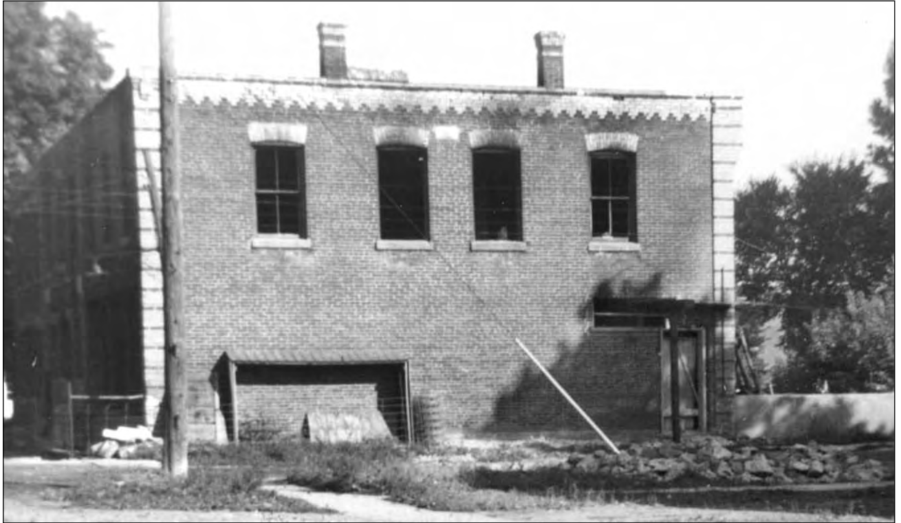
The burnt-out Morrow Farm Equipment building following the fire on May 20, 1951.
