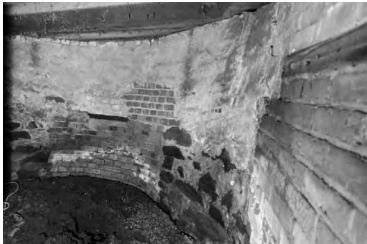
The stone foundation in the "pit" under the main floor shows there have been many repairs over the past 140 years.
