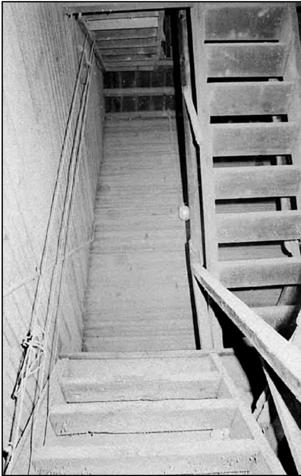
Above: The narrow staircase winds up four storeys to get to the top of the elevator and the cupola.
