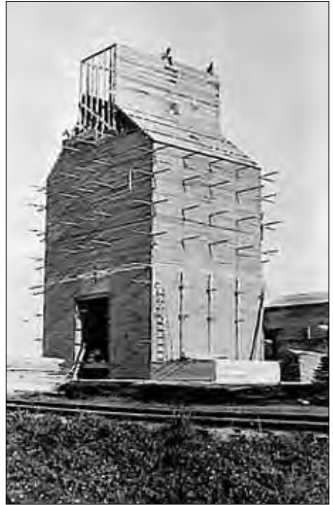
This grain elevator, under construction at Redwood County, Minnesota, in 1910, illustrates the framing of the structure.
