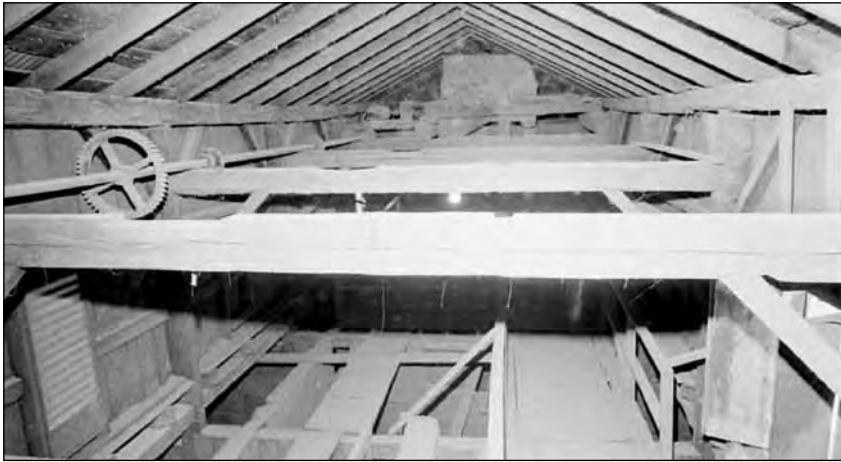
The "headhouse" or "cupola" at the top of the Port Perry elevator.
