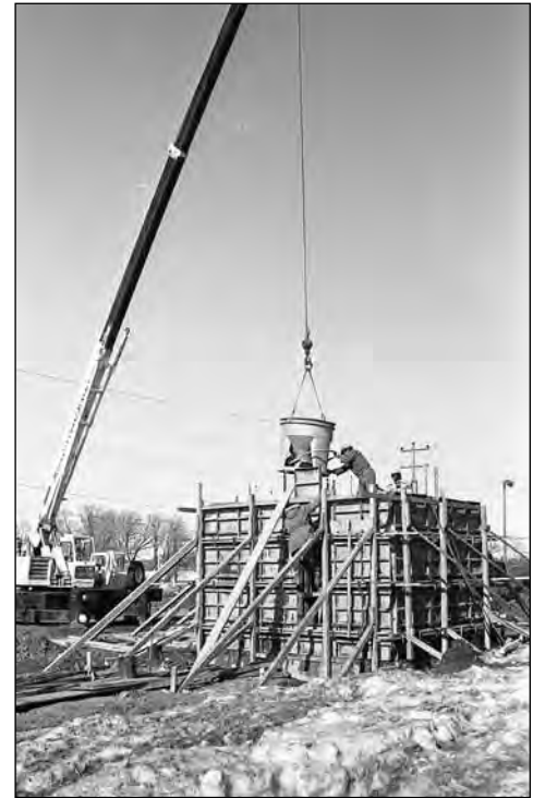
A large crane pours tons of concrete into a form which became the 18" walls of a vault for the Bank of Montreal being built in the Port Perry Plaza in April 1978.
