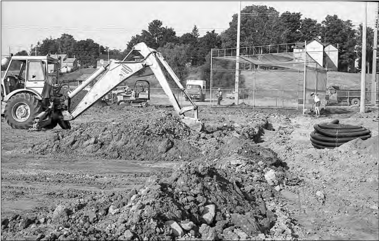
Work was progressing quickly on the long awaited new ball diamond, located on the lakefront at the south end of Palmer Park in July 1973. The new building which will house washrooms and a snack bar is almost completed, and excavations for sewer and water lines are under construction.
