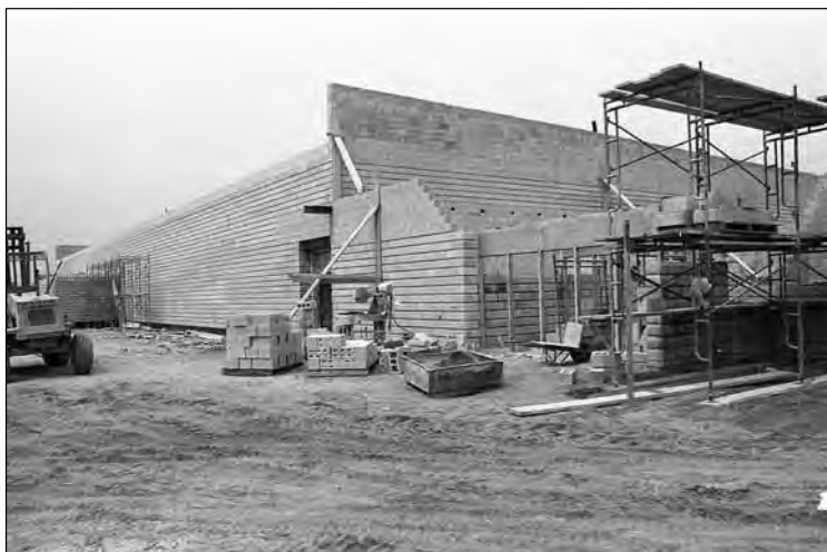
Work on the new Scugog Community Memorial Arena was well underway with the block wall being laid in August 1976.
