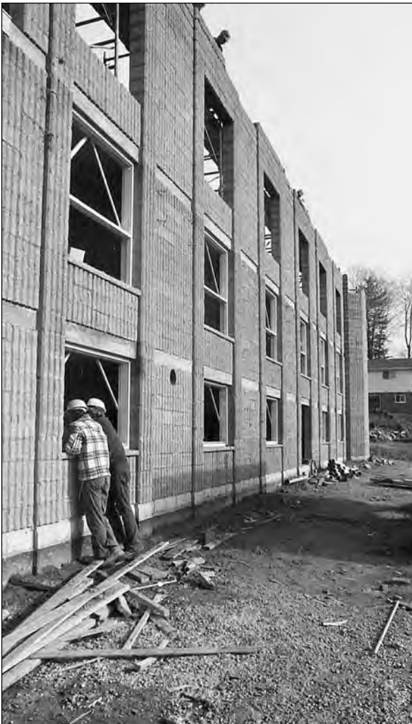
In October 1974, work was underway on the third floor of the new $700,000 Community Memorial Nursing Home in Port Perry. Officials expect it to be completed by March 1975. The home will have 75 beds and greatly expanded support facilities.
