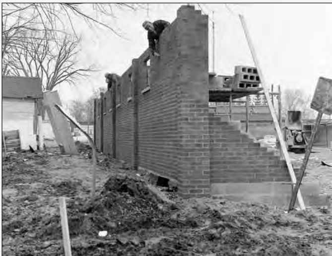
Construction on the new Latcham Centre at the Lake Scugog waterfront was well underway by November 1972. The hall was a gift to the residents of the Village of Port Perry, by Arthur Latcham.
