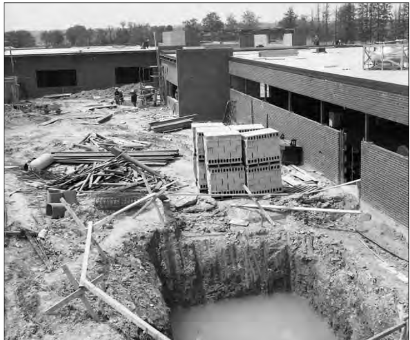
Construction on the new Port Perry Hospital in May 1968. With men, machinery and materials all on site, the contractor was pleased with the progress being made. Completion of the new health facility was completed by the summer of 1969.
