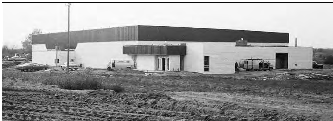
The new Scugog Community Arena was nearing the final stages of construction by October 1976.
