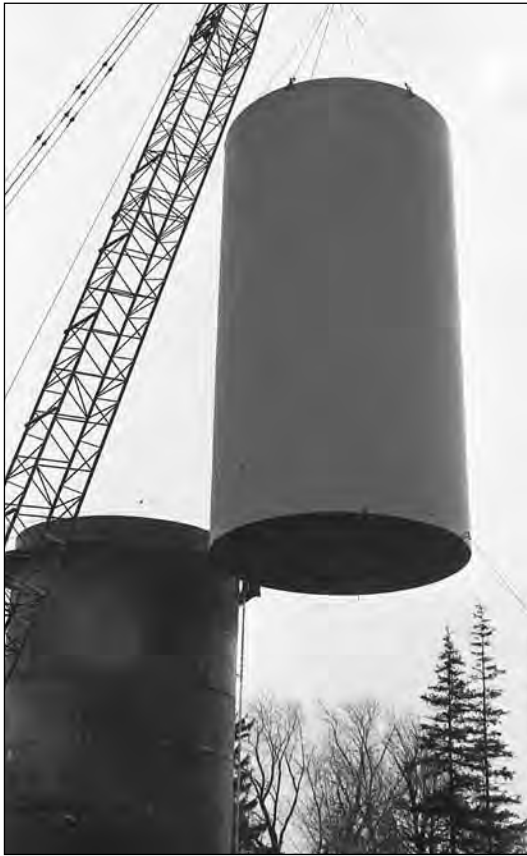
A section of the new Durham Region water tower, located on Silver St., was hoisted into place by a crane in May 1979.
