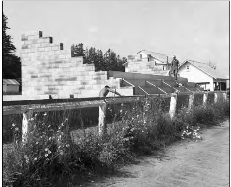
Work on the new grandstand at the fairgrounds was progressing smoothly by July 1967. The fair board expects the construction will be completed in time for the fall fair. Mel-Ron Construction was awarded the contract and when it is completed, the grandstand will seat about 600 people.
