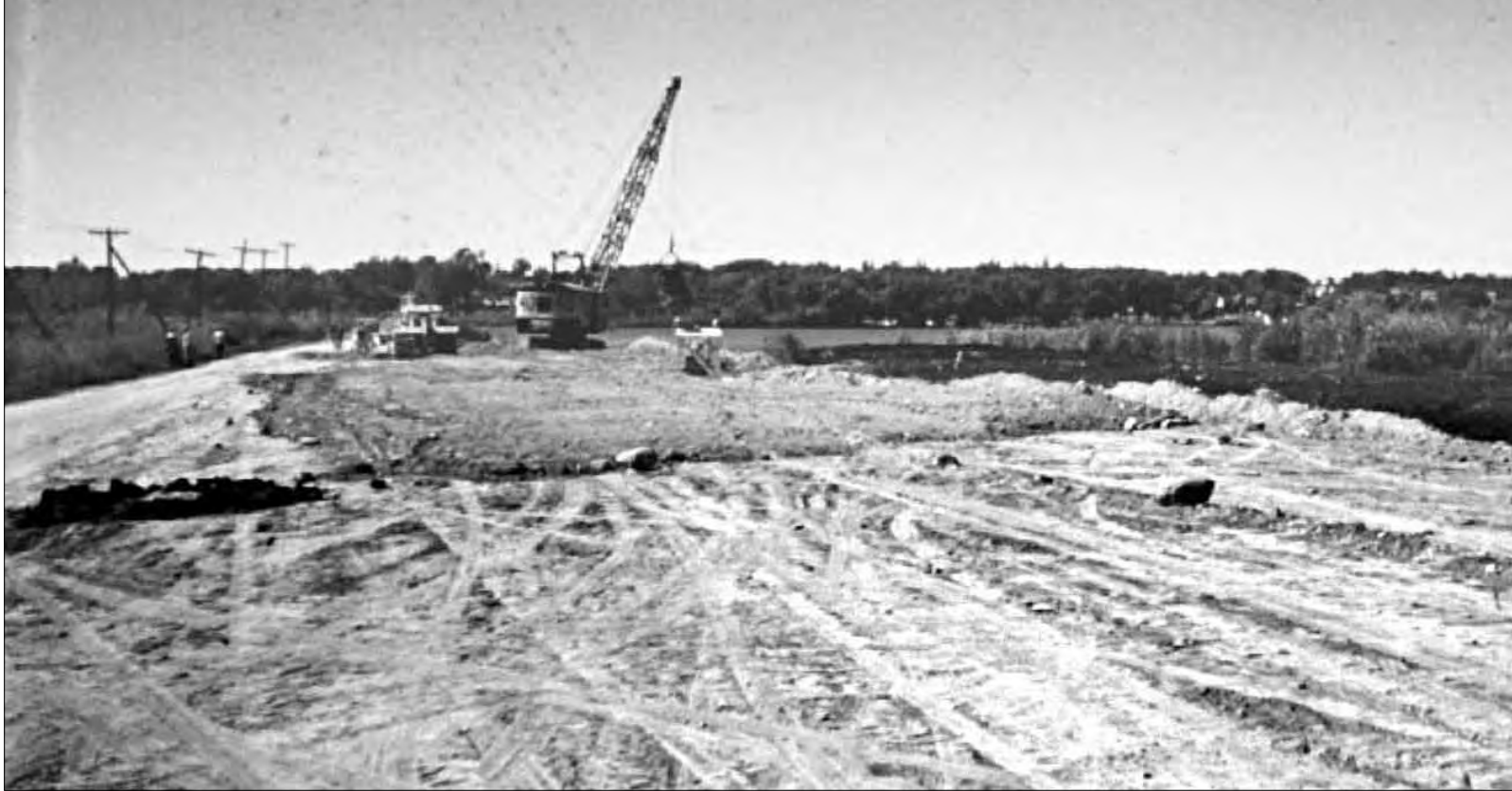
Photo at left, flooded causeway in the years before reconstruction. Above and below, work underway on widening the causeway in 1960.
