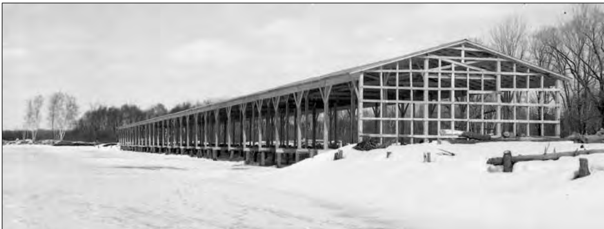
Phil Goreski, owner of Club Annrene, has been busy during the winter erecting two large covered boat slips. The buildings will be two of the largest of their type to be built on a man-made canal and will hold about 62 boats. The slips are designed by Mr. Goreski, with the largest measuring 410'x28' and the other 390'x24'. Photo taken April 1970.
