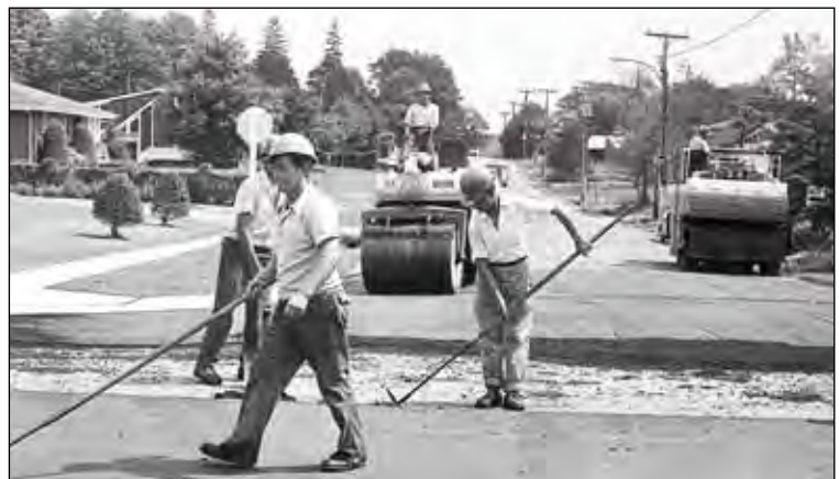
Work crews finished off the final topping of asphalt on the contentious Lilla Street widening project, paving from Hwy. 7A to the north limits of town. They are seen here doing a section near the intersection with Kent Street.
