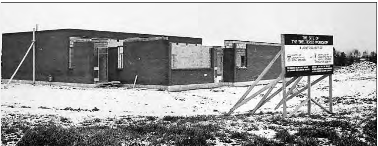
Construction was well underway on the Central Seven workshop for mentally handicapped adults in December 1978.
