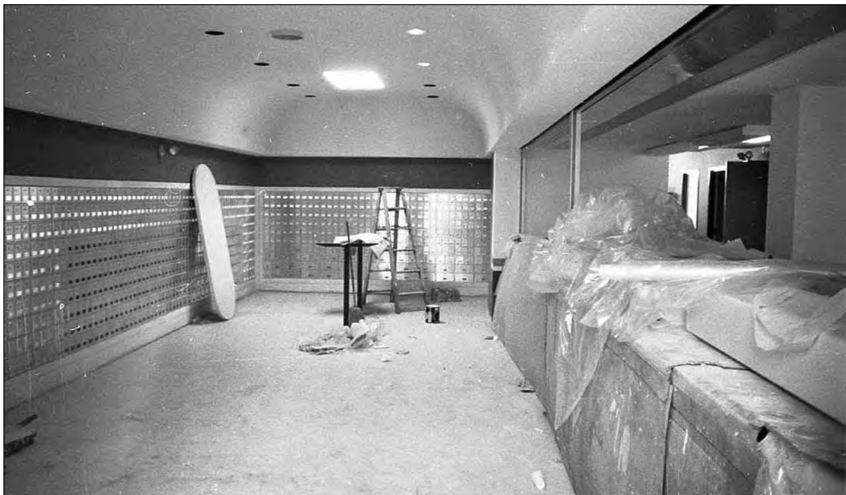
Renovations on the interior of the Post Office in March 1975, when the lobby and service area underwent a complete upgrading.
